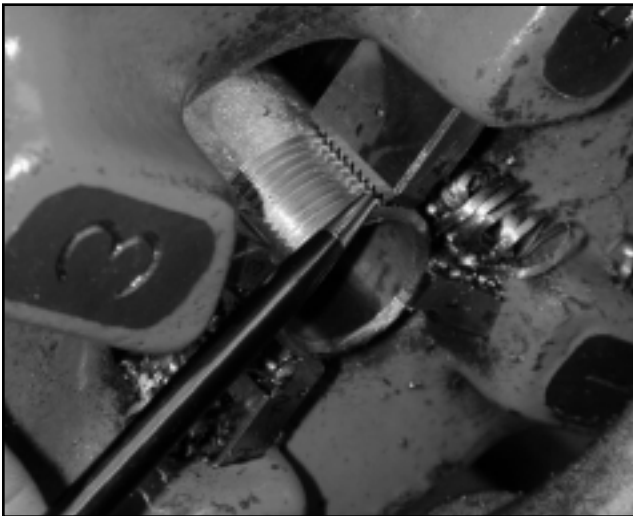
Figure 9: When proper thread length is achieved the end of the conduit becomes flush with the ends of the die segments. (Courtesy of Wheatland Tube)
